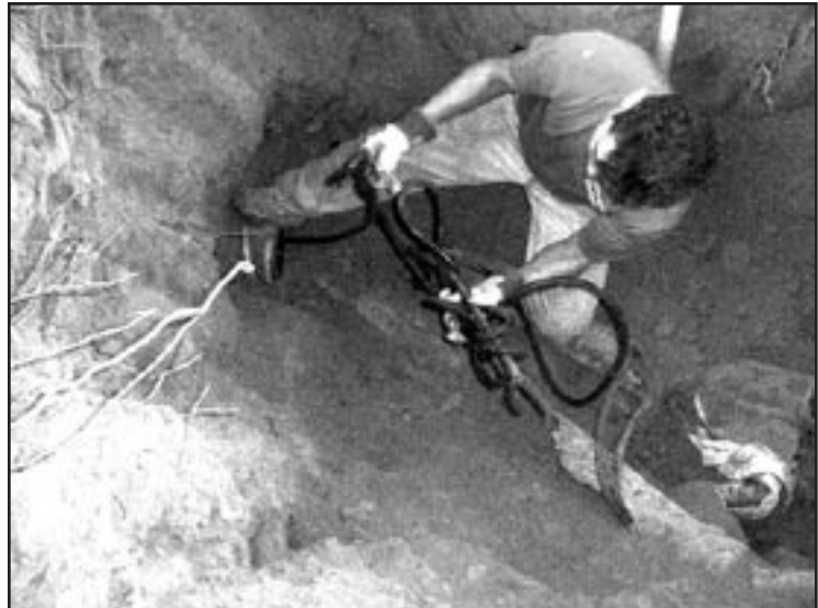
Worker dude inserts video camera into sewer pipe to view problem on the monitor
